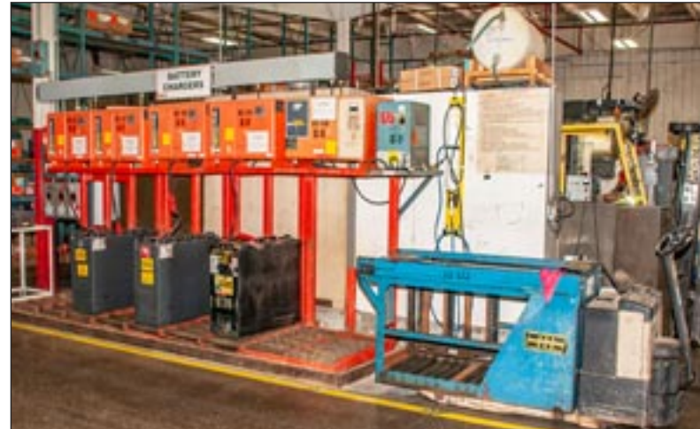
BATTERY CHARGING STATION
