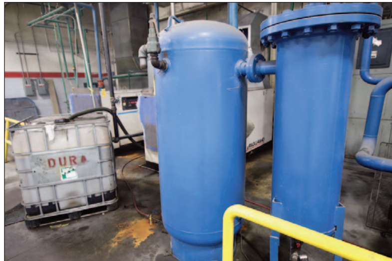
200 GALLON RECEIVER TANK
