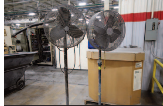
FLOOR AND WALL FANS
